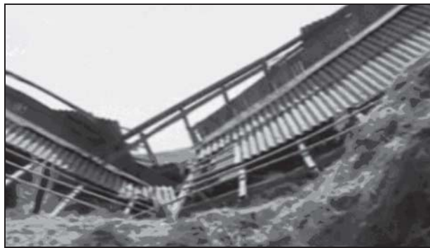
Fig. 2. The DI - Barn that has the supporting walls collapsed
