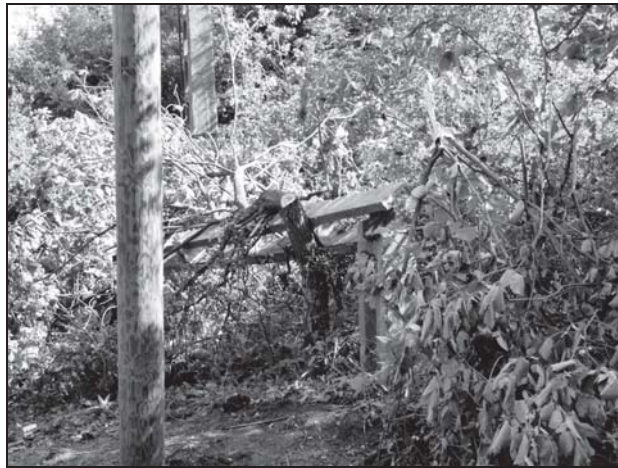
Fig. 5. The fifth DI - Broken electrical transmission lines
