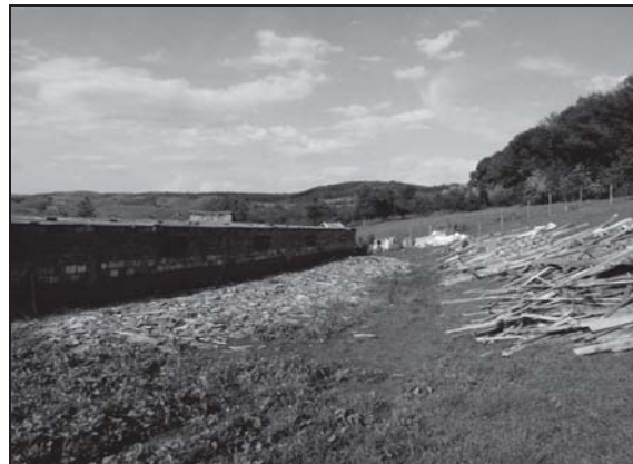
Fig. 4. The Third DI – Uplift of roof structure of an stable
