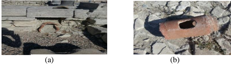
Fig. 2. (a) Round terracotta pipe installed under the floor possibly carrying storm-water and (b) Terracotta pipe with inspection aperture from Amathus.
