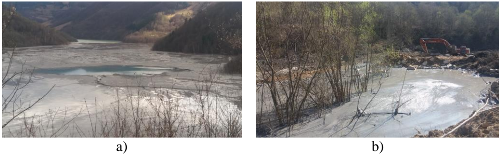
Fig. 2. Valea Şesii tailing pond: a) internal suffusion cone in the stabilized area; b) temporary works downstream of dam to contain the pollution event (source: Ciungan, C., 2017)
